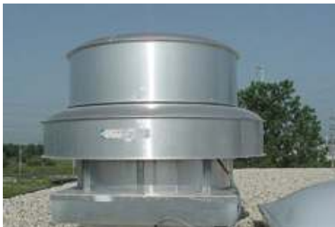
Air handlers on roof of D.L.S.
